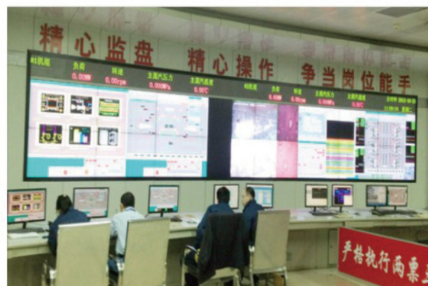
常州电厂 Changzhou Power Plant
